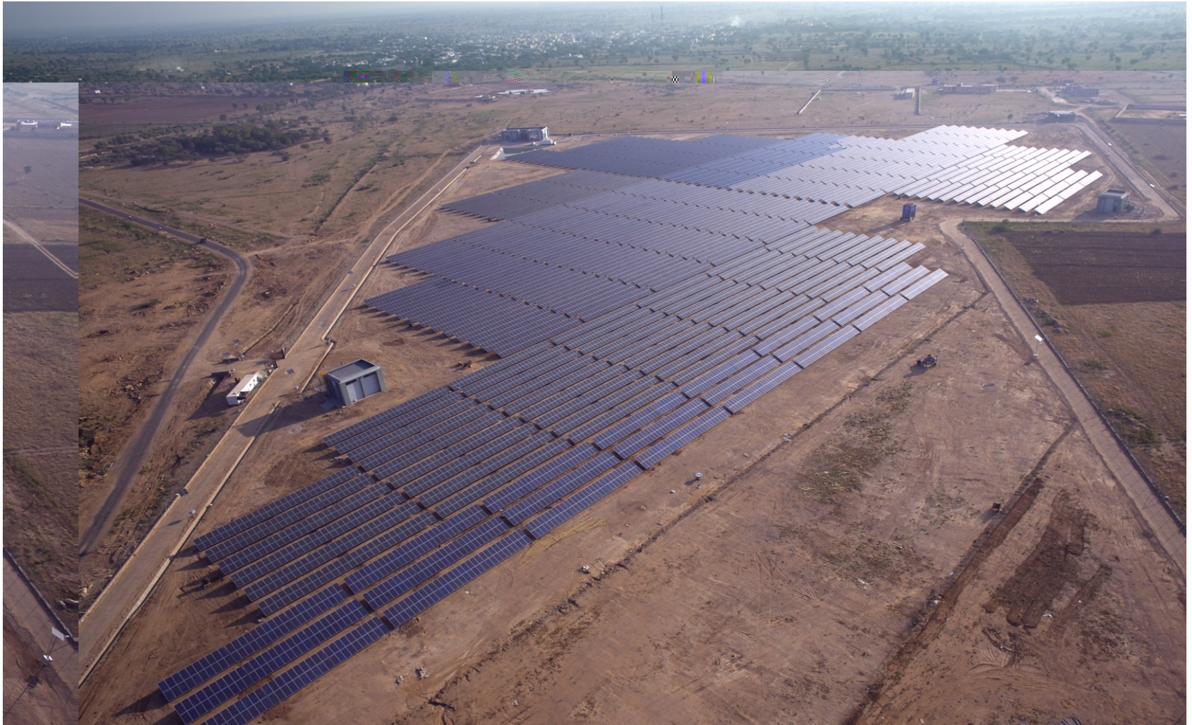
5 MWp PV (Crystalline) Grid Power Plant at Khimsar Vllage, Jodhpur, Rajasthan
